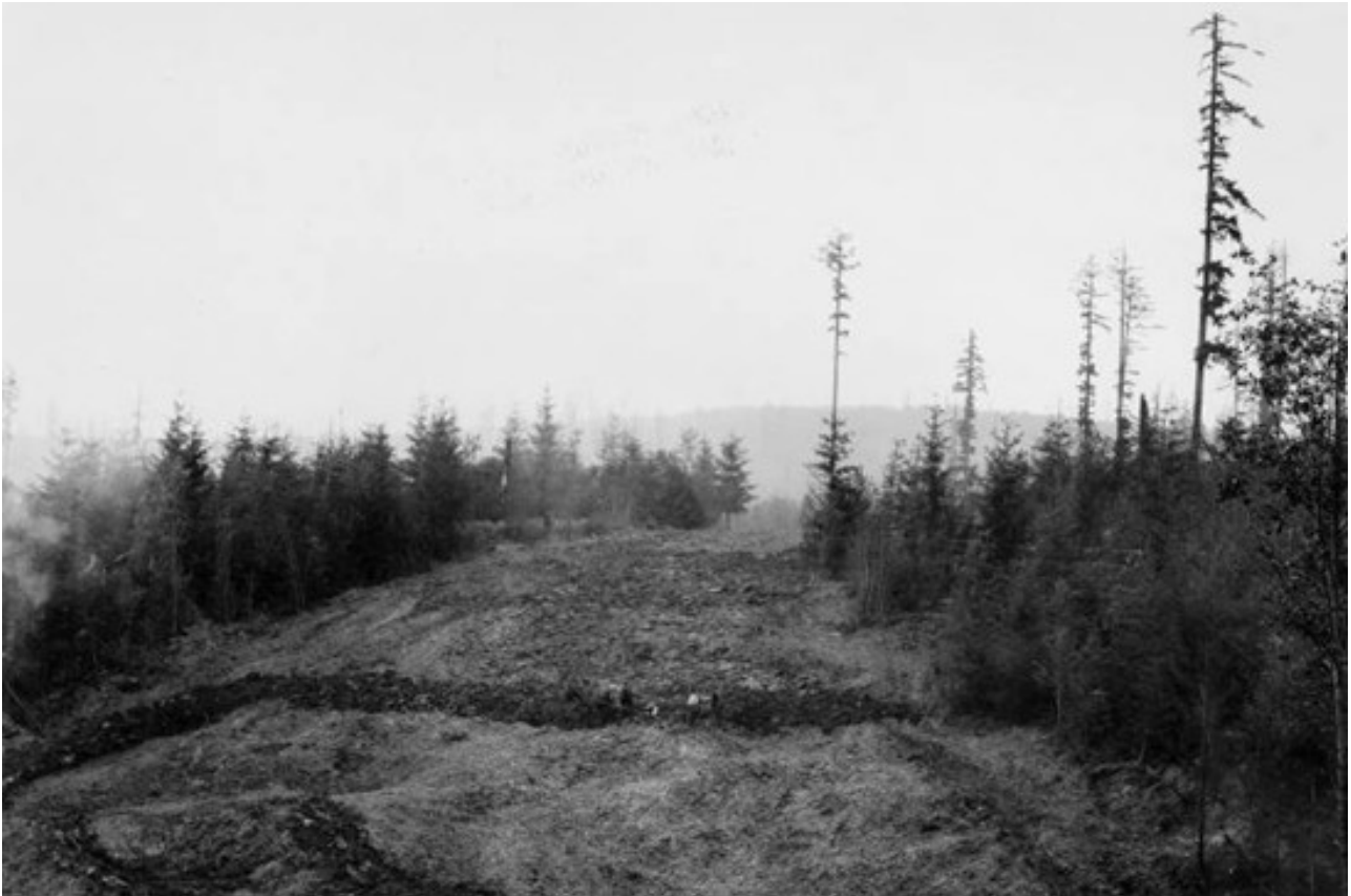
Longview CC's new course under construction. Horse team in center- 5-25-1926 (courtesy of Longview Public Library).
